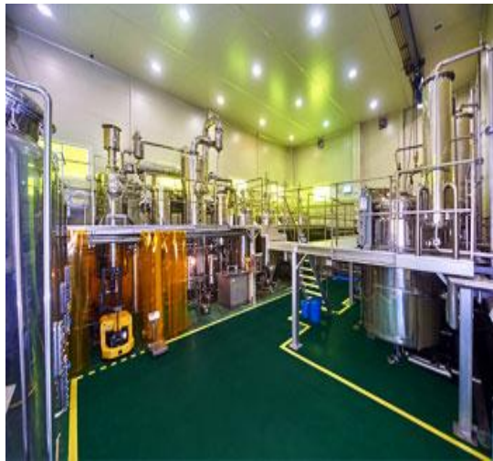
EXTRACTION & CONCENTRATION FACILITY
