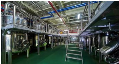
MIXING AND EXTRACTION TANK
